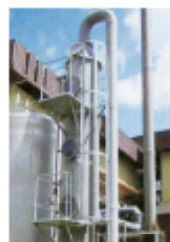
Vertical Packed Tower Gas Scrubbers
